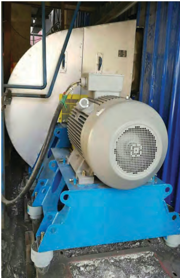
Clinker fan installed close to clinker cooler wall.
