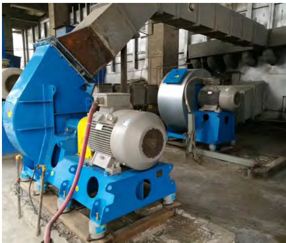
Group of cooler fans installed and anti-vibration mounts with new foundations.
